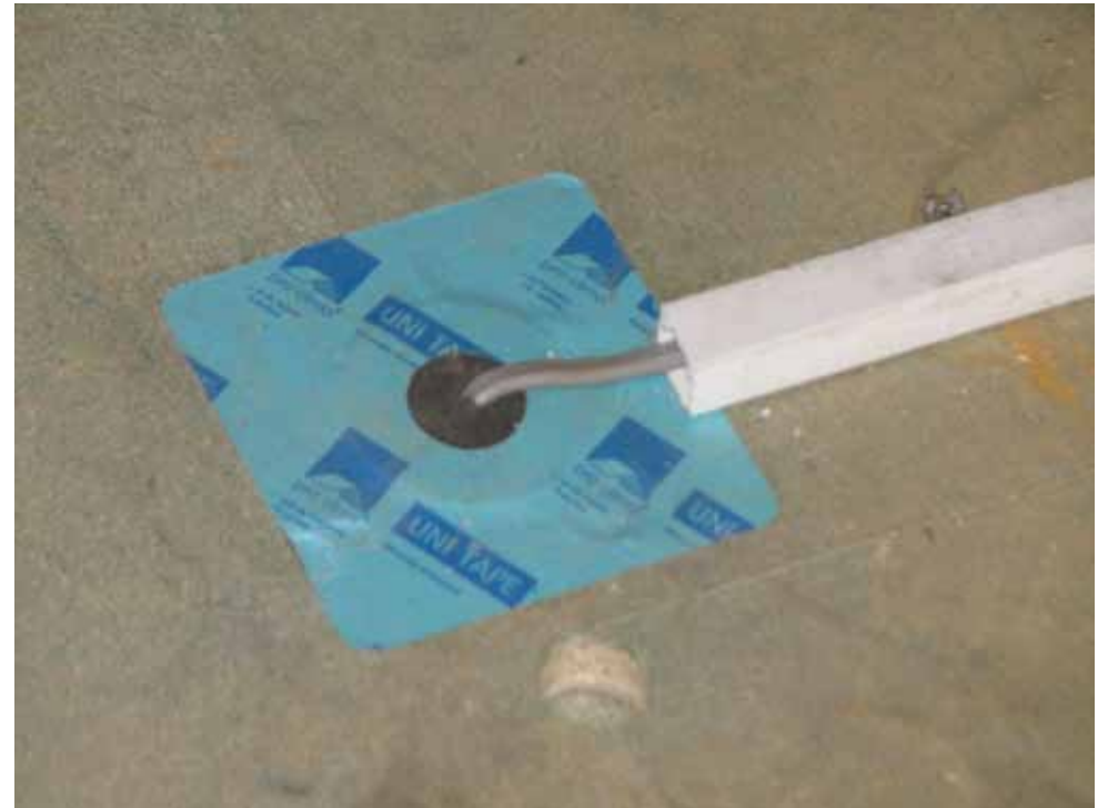
The boards allowed access to be maintained in the roof space and simple seals to be used around services
