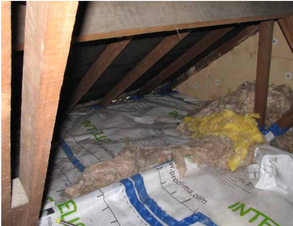
A continuous membrane installed in the loft at Passfield Drive to create the airtightness barrier, sealed to the external walls.
