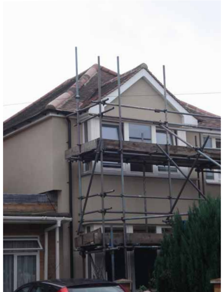
Awaiting scaffolding removal following completion of render - final air testing to be completed
