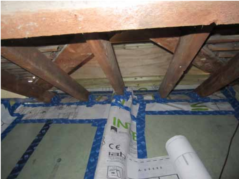
18mm OSB provides the airtight barrier. Membranes are used to seal around roof timbers and connect to the external walls
