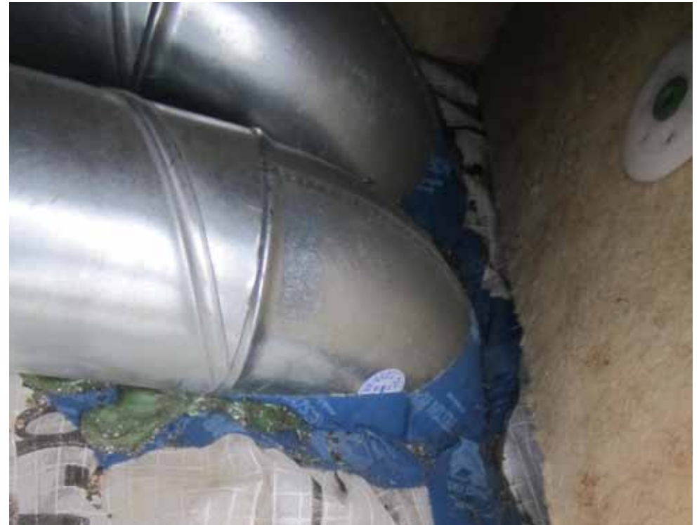
The membrane proved difficult to install; requiring many taped joints and difficult sealing details around service penetrations
